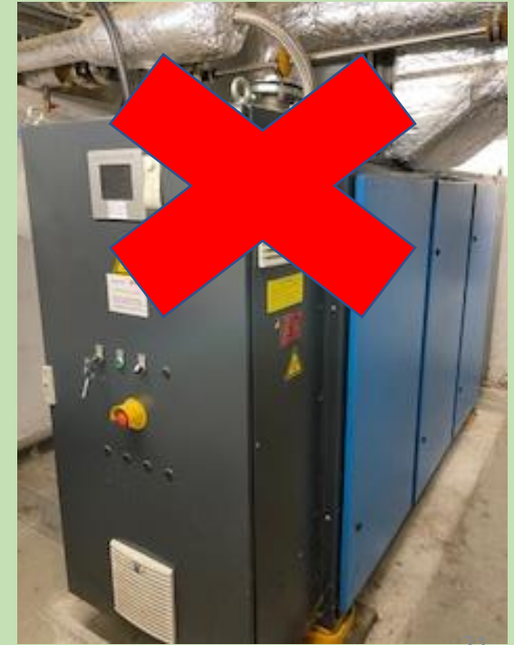
Leistung : 50 kw el. / 80 kw therm.
