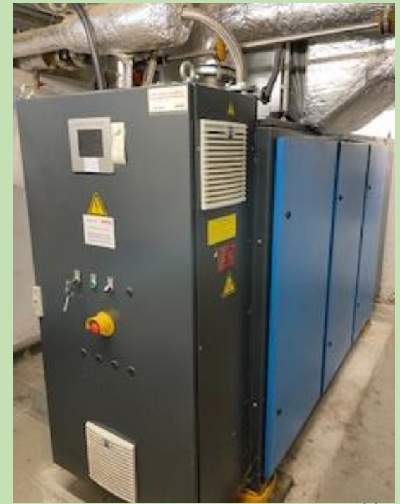
Leistung : 50 kw el. / 80 kw therm.
